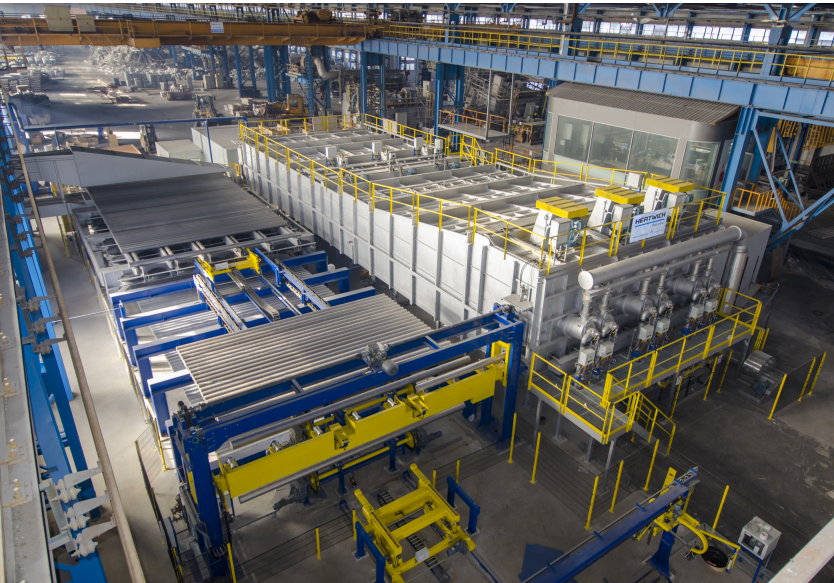
Continuous Homogenizing Plant at Eti Alüminyum A.S., Turkey
