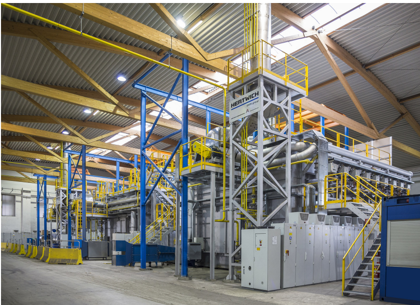
Batch Homogenizing Plant at AMAG, Ranshofen
