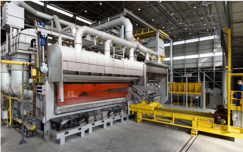
Hertwich Ecomelt-PS200 with rail-guided skimming machine at Hydro Ghlin
