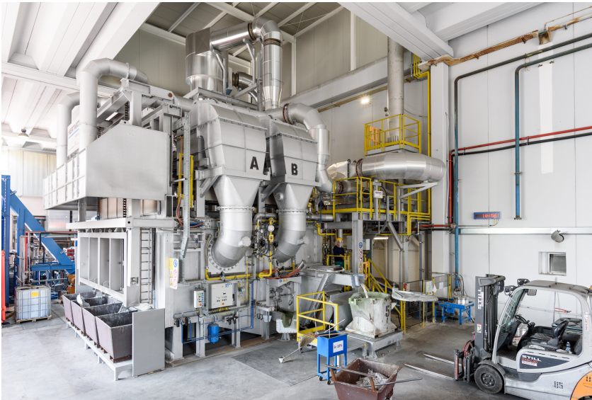
Hertwich chip melting furnace at Cromodora, Italy
